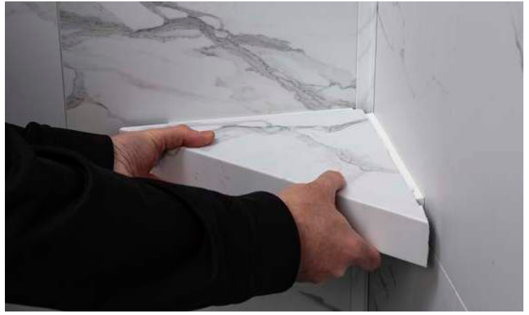
Continue to push the shelf into place for a tight fit against the wall.
