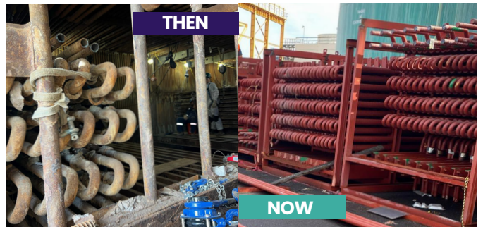
Waterwall and Economizer Elements (Unit 3, Palo Seco).
